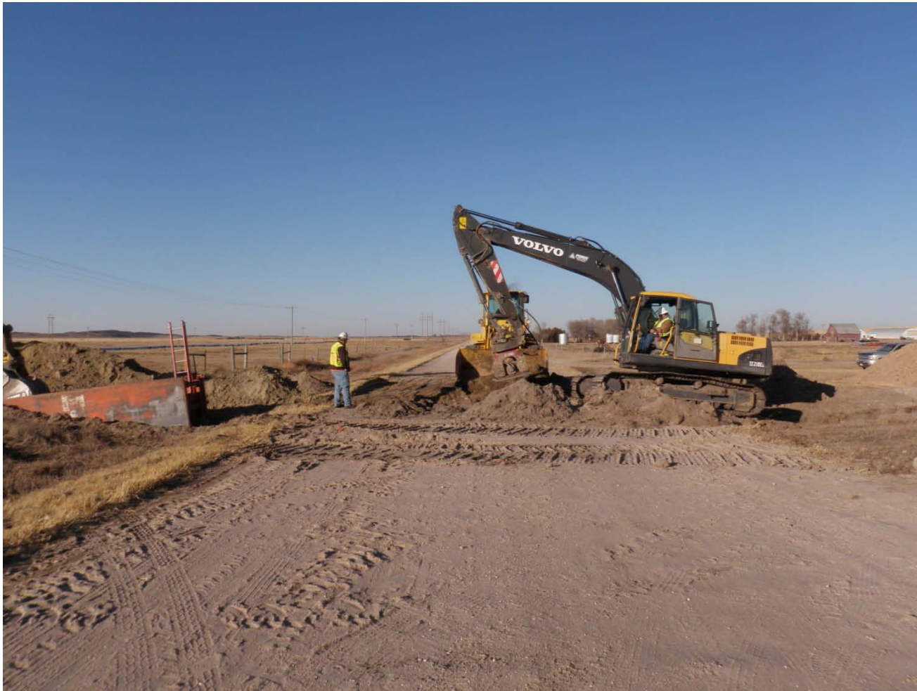
Sessions compacting backfill over PVC line A8 at County Road RR crossing.
