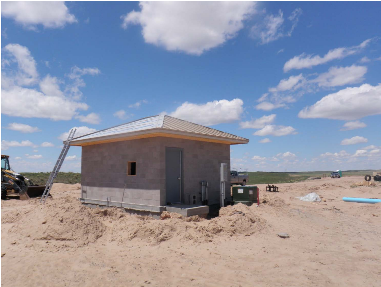
Completed control building at collection tank site.
