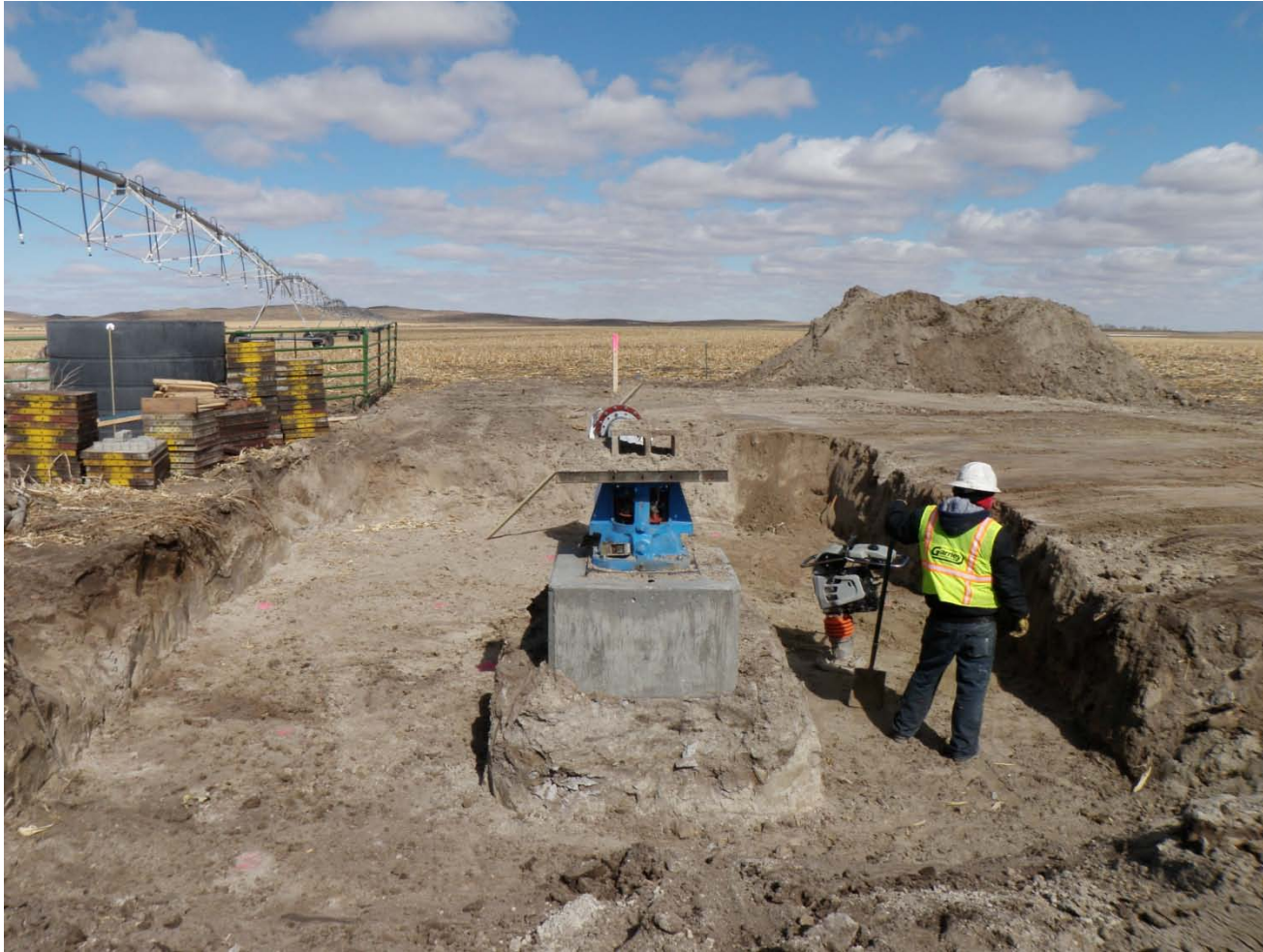
Garney preparing ground to set footing forms for well house at site A3.
