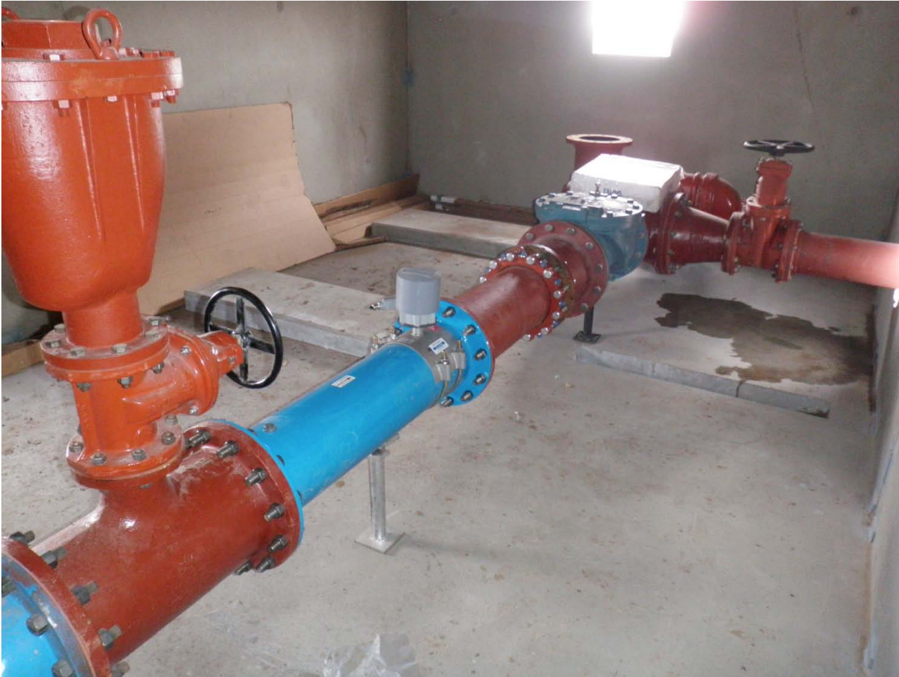
Well house piping, showing air valve and irrigation pipe stub.
