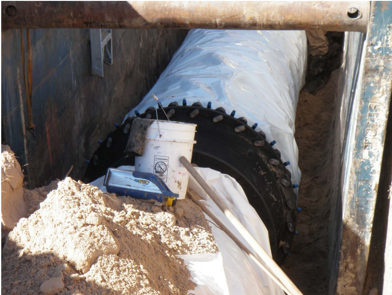
View of 42"x36" reducer at Station 442+60 on main transmission pipeline.
