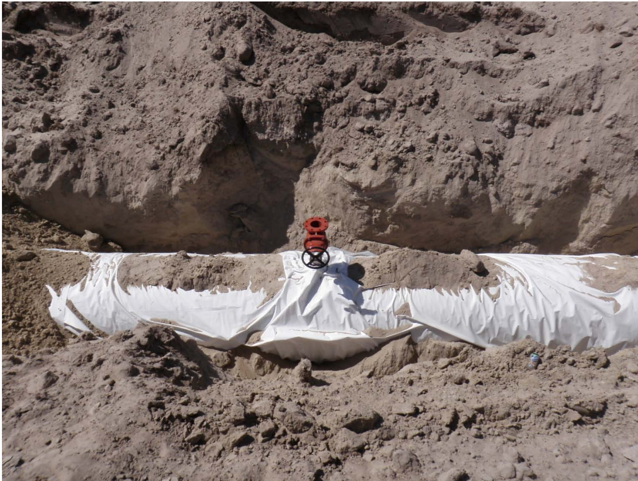
Air release on main pipeline installed at approximately Station 607+05.
