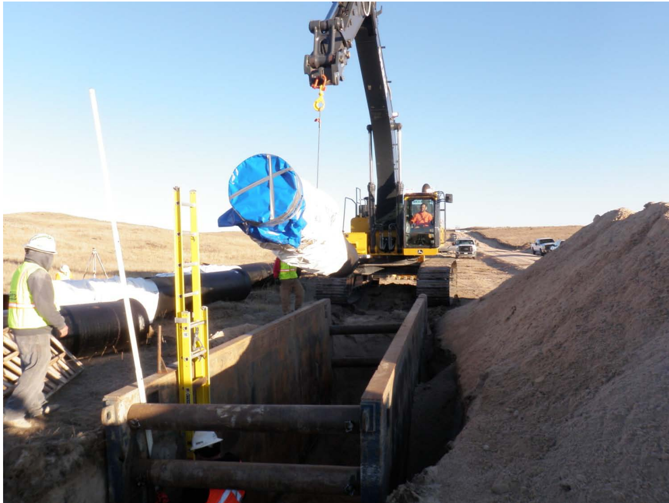
Garney placing first stick of ductile iron pipe in the ground at Station 9+68.
