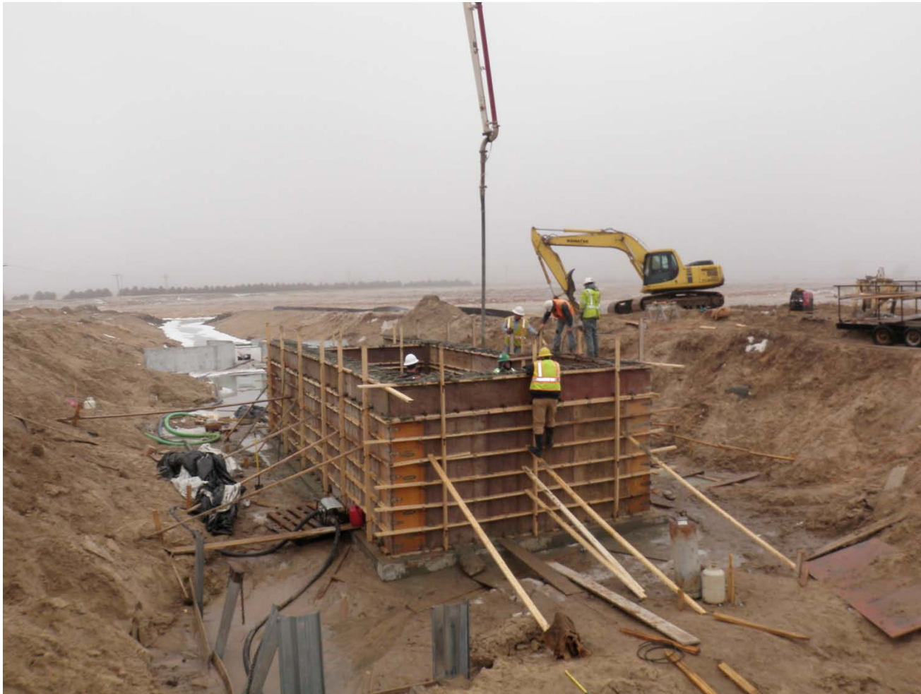
Sessions working on concrete placement in the walls of the outfall structure.
