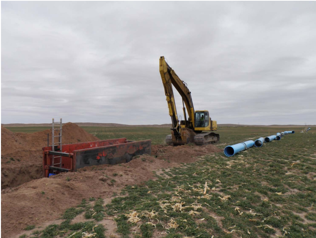
Sessions excavating trench for installation of PVC pipe on collection line A5.
