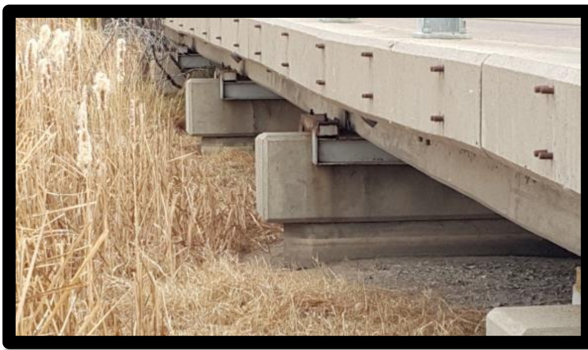
Photo 5: Highway 385 Bridge – silt and cattails have reduced clearance from 8+ feet to 3-4 feet
